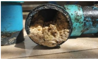
Clogged Drainage Pipe
